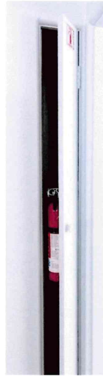
fire extinguisher closet in kitchen
